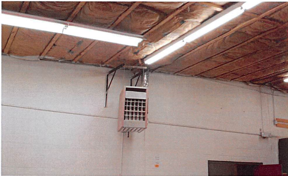
Interior-Reznor heater in warehouse area
